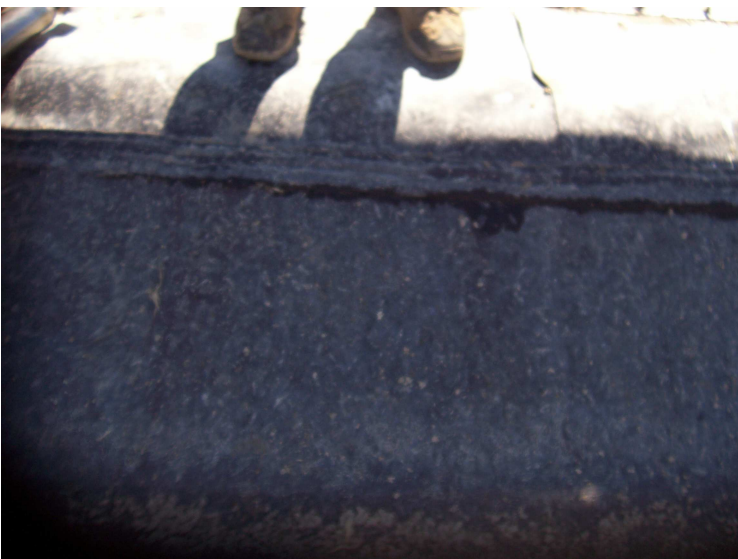
Seepage showing along concrete/Poly-Lock interface from back-water pressure.
