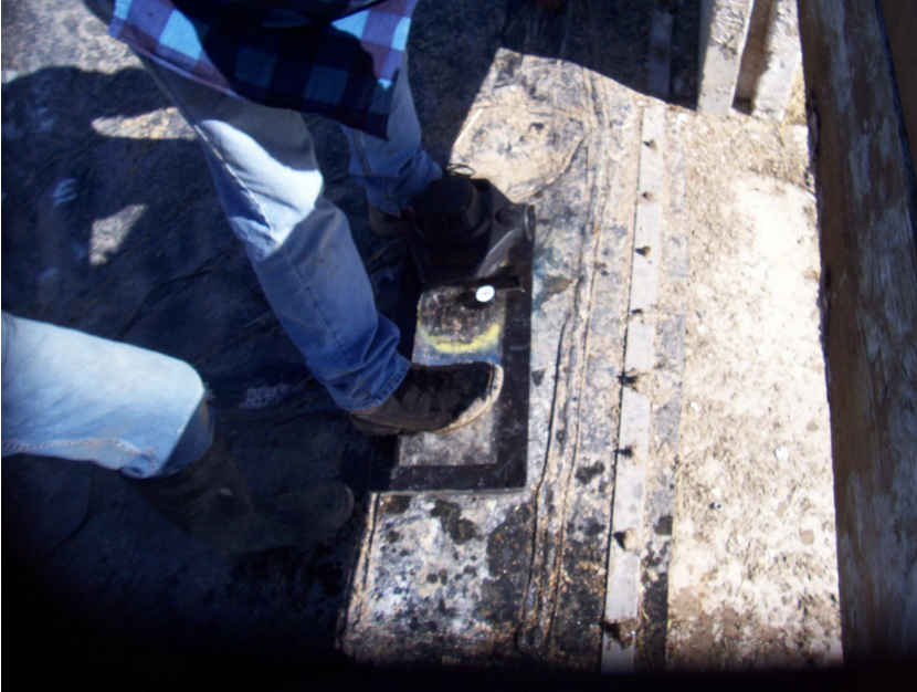
Vacuum testing patch along west wall of aeration pump section where 3 leaks were found with v.box testing.
