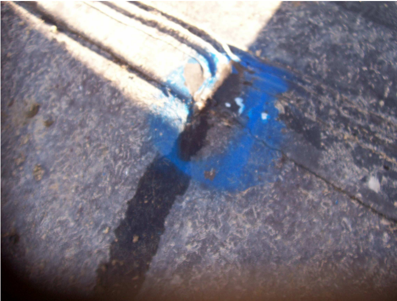
Seep at previously repaired Poly-Lock joint attachment at concrete slope in aeration pump section.
