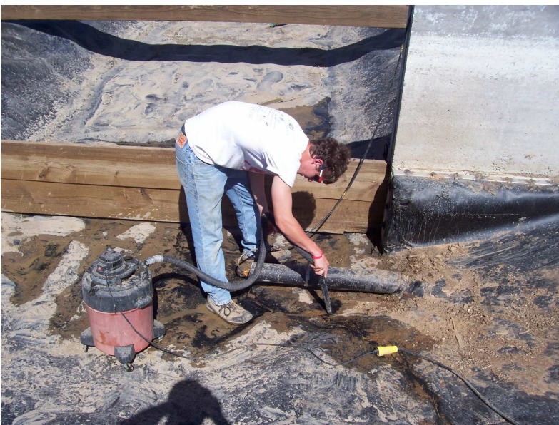
Middle low section of south side of raceway being water tested for leaks. Two holes found.
