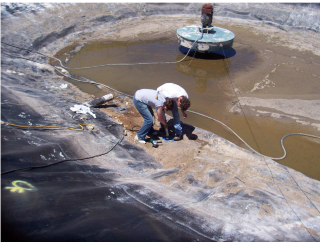
Two holes discovered in liner at aeration pump section properly repaired to be leak free by v.box testing. Water behind liner revealing leaks was pumped out in advance of heat seam repair.
