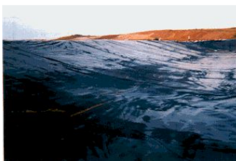
Figure 5b - Same Retention Pond Liner on Cold Morning With Minor Bridging at Toe of Slope
