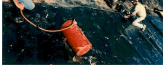
Figure 8 - Consider the patching frequency required when air pressure testing panel widths at the toes of slopes. Can this really be the best practice?
